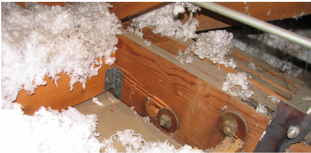
Photo #4. Row tear-out of bottom chord at splice connection.
