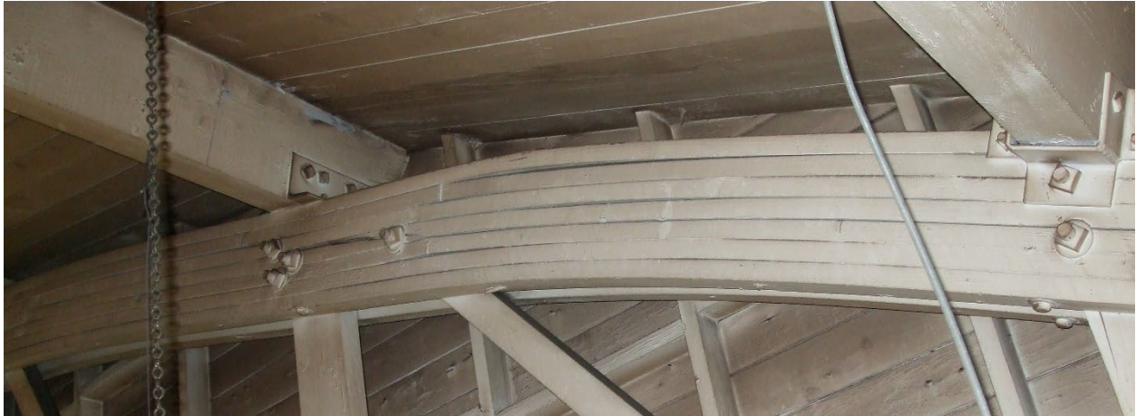
Photo #2. Top chord showing effects of adhesive deterioration
