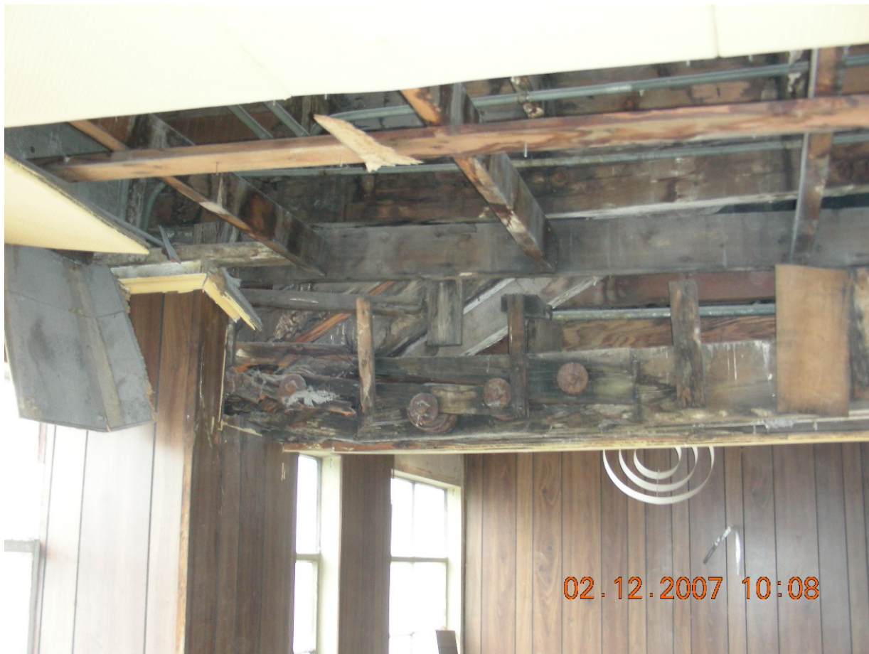
Photo #6 Decayed heel caused by poor roof drainage Note the water staining on the members.
