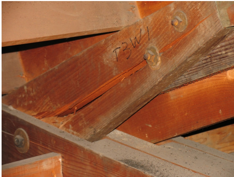
Photo #3. Top Chord failure at truss heel.
