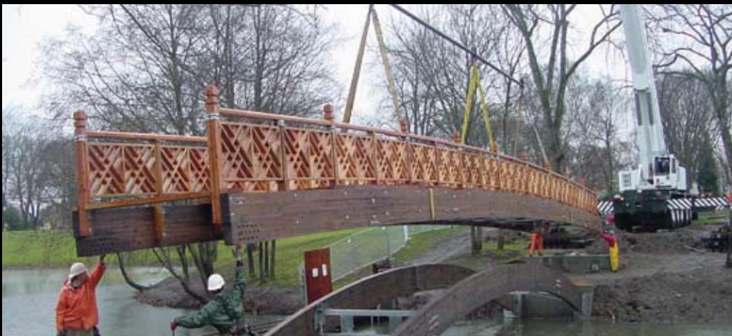
A 7' x 100' arch-under bridge in Washington was assembled at Western Wood Structures, then shipped to the site, where a crane was employed to facilitate the installation. (See cover photo for completed bridge).
