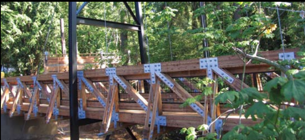
The 8' x 106' timber suspension bridge at The Oregon Zoo enhances the natural setting.
