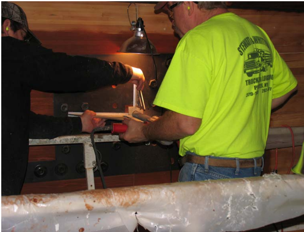
Figure 12. Cutting the “Z” hanger in half with rebar cutting bit. The workman on the left is using two framing squares to align the drill bit. It took just over an hour to core through the ½” x 10” back plate of the “Z” hanger.
