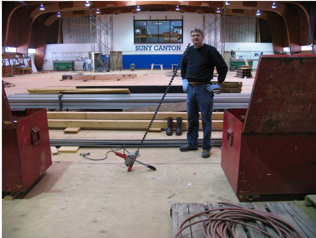
Figure 10. WWSI jobsite superintendent, Ray Kennedy with 54 inch drill bit used to drill for epoxy dowels.
