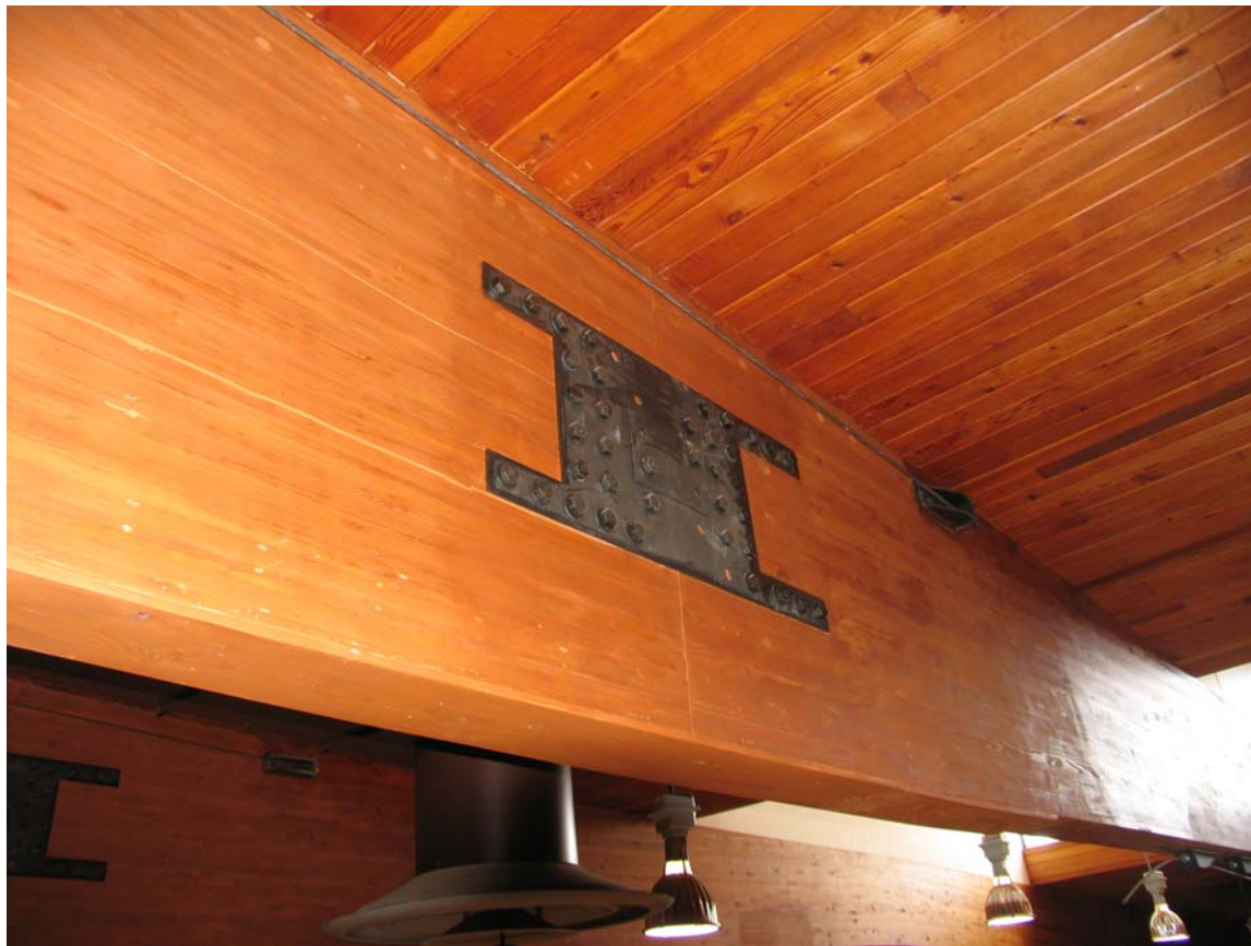
Figure 9. Steel side plates used to transfer reaction from center beam to arch section. The paste type of epoxy used to seal the member at the original split does not receive the stain and can be seen as a light line at the bottom of the plate. The post tensioning cable for the top plate is seen next to the timber decking.
