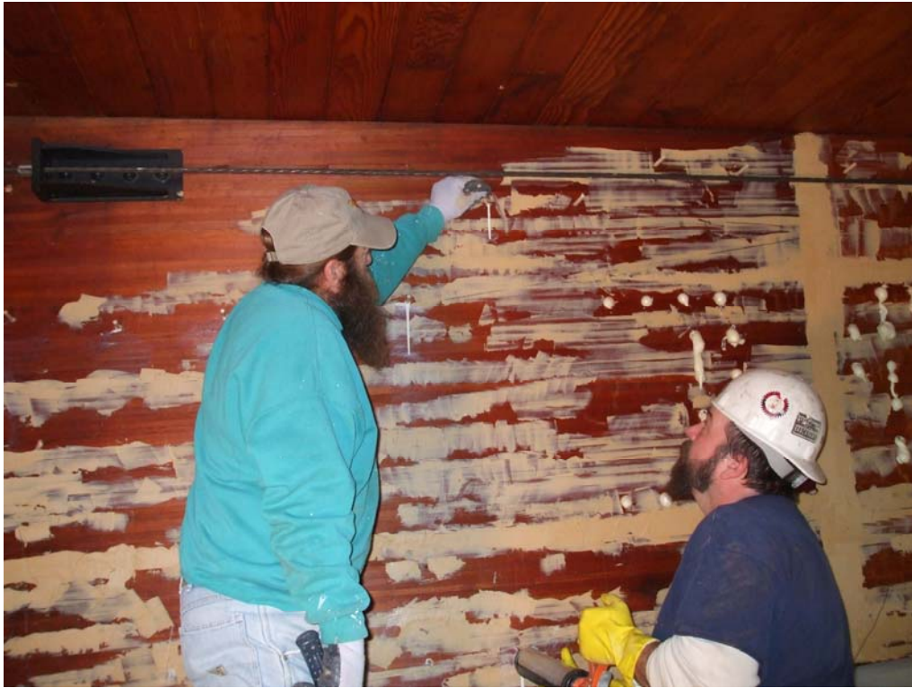
Figure 11. Workmen pump epoxy into arch member. The member is completely sealed to prevent the epoxy from leaking while allowing the epoxy to fill all of the voids in the member.
